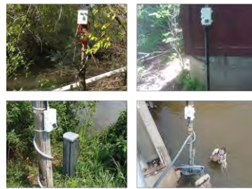
Figure 3.6 Examples of Telemetry Unit Mounting Configurations at Stream Monitoring Sites
