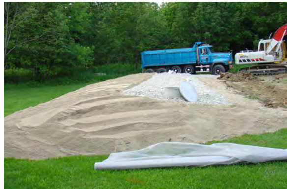
There are several different types of POWTS including at-grade, conventional systems, constructed-wetland, dripline, in-ground pressure, mound systems, and holding tank systems. A mound system is pictured here.
